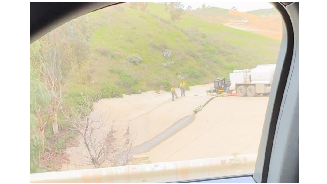
Photograph 4 (March 16, 2024 Complaint, COMP-60321) Photograph showing active pumping and discharge from either the south detention basin or the vacuum truck.
